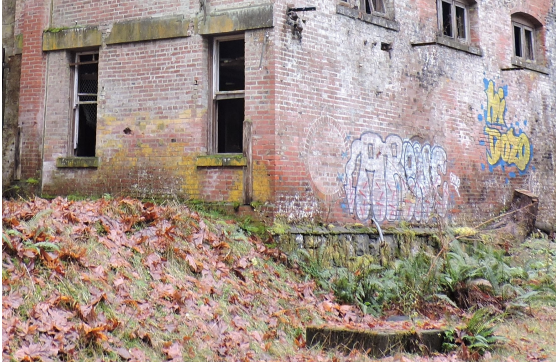
NE corner, showing build up of earth along front side
