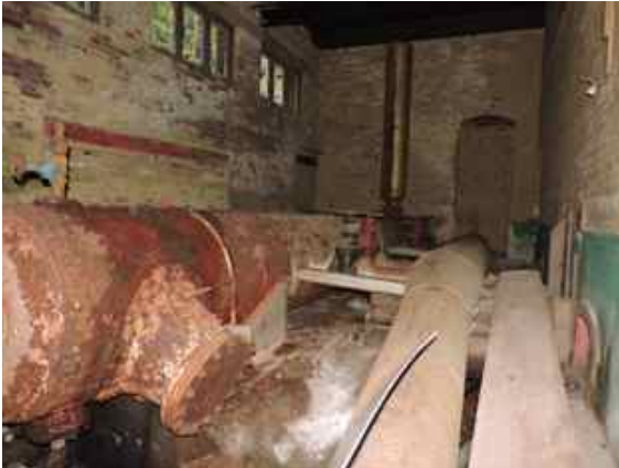
Interior of SW side addition, still housing massive power generation equipment seen outdoors in 1898 photographs of original building
