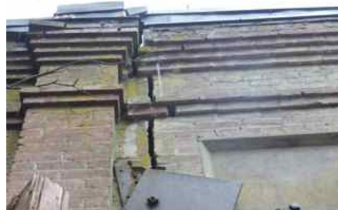
Cracking at junction between 1898 original structure and 1901 NE side addition
