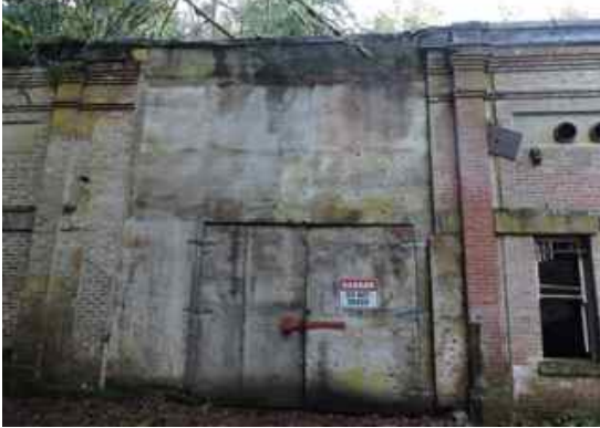
Front facade, note missing masonry front of 1898 structure.
