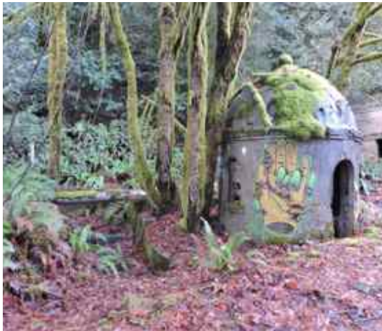
Expansion Bell; note trees that have grown adjacent to the structure and build up of soil
