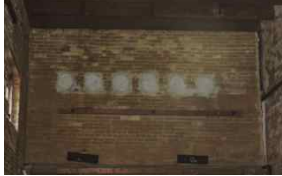
Sealed tubes on front wall of NE side addition, used as exits for transmission lines.
