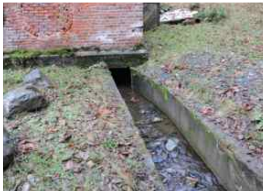
Tailrace from NW rear corner of Powerhouse
