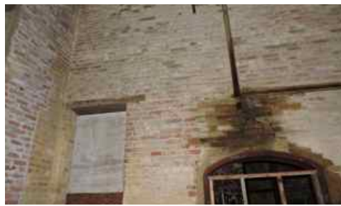
SE corner of central area; note staining on masonry, reinforcement near ceiling, and blocked doorway to SW side addition.
