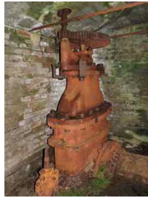
Water control valve (Pelton?)
