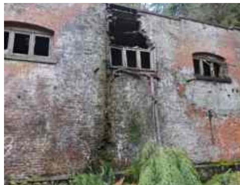
NE facade damage from tree growth
