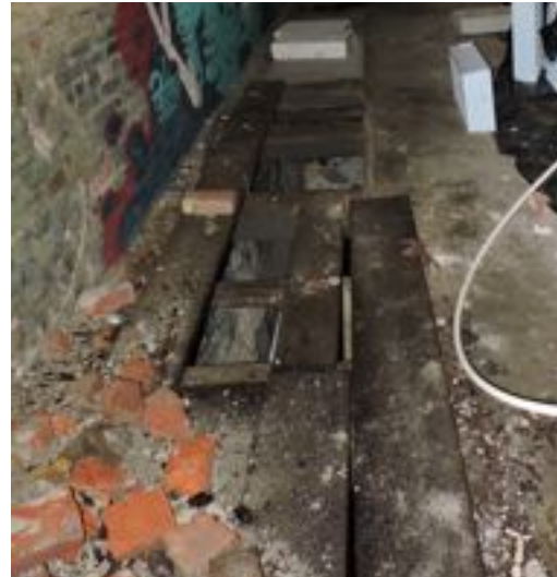
Damaged floor near rear entrance
