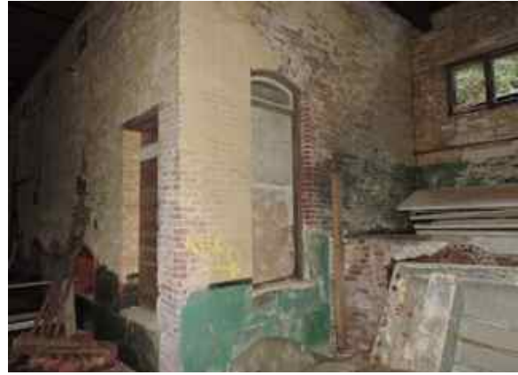
Walls of the SW side addition, taken from back of central area. Note blocked doorway and window providing access and view the enclosed area.
