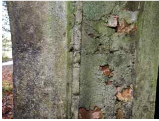
Side view of Expansion Bell doorway providing a sense of wall thickness
