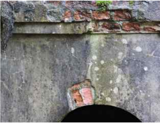
Damage to concrete skin of Expansion Bell
