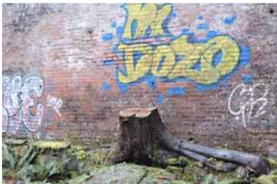
NE facade tree roots in foundation
