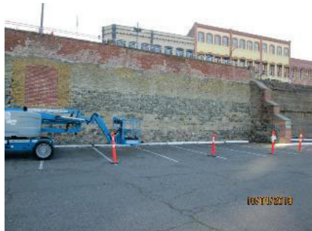
PHOTO 27: Current (2018) overview of southerly section of wall. Poorly executed re-pointing and filling of the old beam pockets is evident.
