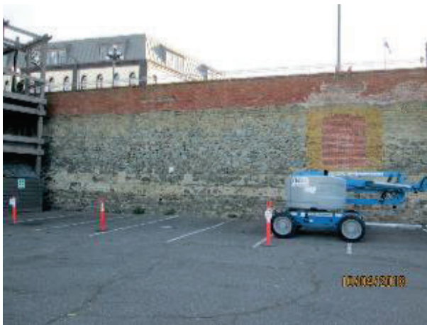
PHOTO 26: Current (2018) overview of northerly section of wall. Some poorly executed re-pointing of the upper section of brick work is evident.
