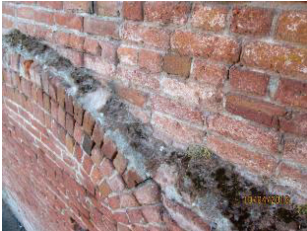
PHOTO 75: The original mortar droppings are clearly visible on this set back ledge. Organic material deposits and growth further act to retain water in high wind and rain events.
