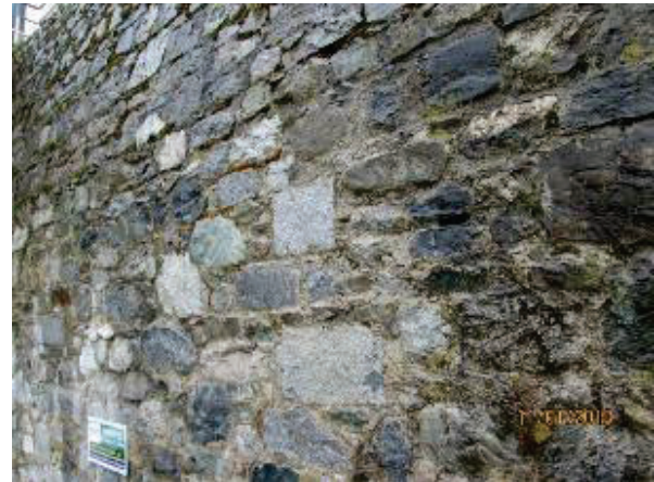
PHOTO 85: A distinct drainage and wetting pattern to the surface of the wall was observed during a recent high rain event.
