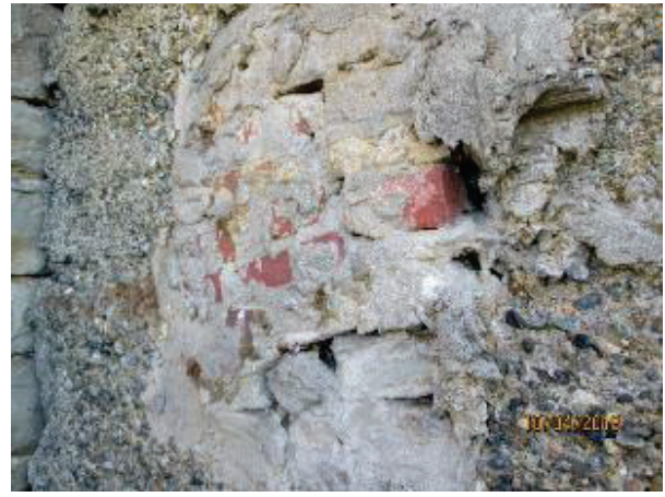
PHOTO 67: poorly executed patch repair. This repair predates the 2008 photos and appears as a lighter patch in PHOTO 18, taken in the early 1970's
