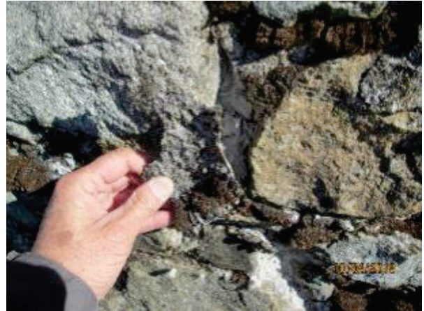
PHOTO 81: Loose stonework. Several of the smaller stone filler pieces where coursing and levelling occurred during construction are now loose or debonded from the wall.
