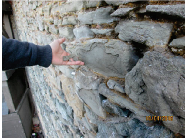
PHOTO 36: Exfoliation of the Sandstone surface is clearly evident
