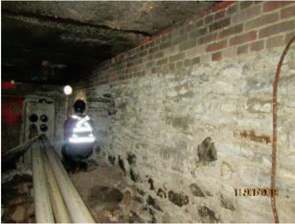
PHOTO 55: Looking south, access to the full extent of the chamber is blocked by a precast concrete vault.
