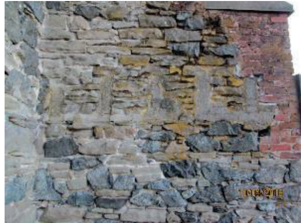
PHOTO 42: Former floor joist pockets have been filled with cementitious material
