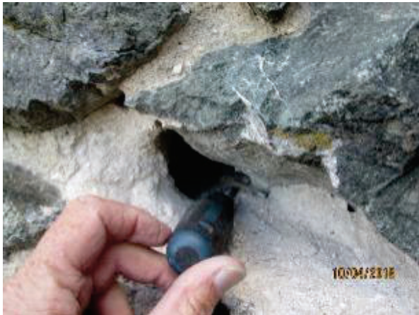
PHOTO 34: Large void in mortar joint
