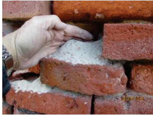
PHOTO 76: The friable nature of the decayed mortar, simply demonstrated. The burnt lime that provides the material stability has been lost due fresh water leaching.
