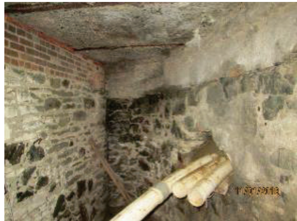
PHOTO 54: The northerly intersection between the stone retaining wall and the exterior wall of the old warehouse.
