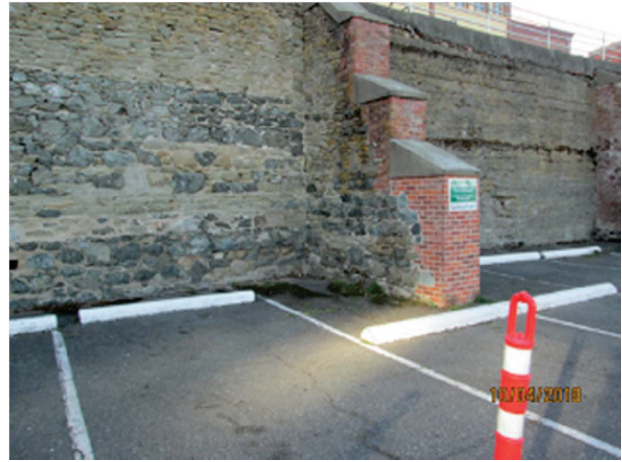
PHOTO 40: Current condition of the wall. Repaired using a mixture of recycled and modern clay bricks.
