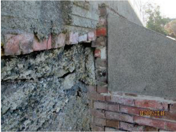
PHOTO 68: Poor condition of the upper and presumably later layers of concrete that form the current sidewalk curb.
