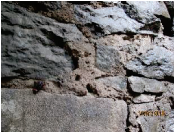
PHOTO 61: A close up of the easterly side stone retaining wall. The mortar joints appear to be in good unweathered condition.
