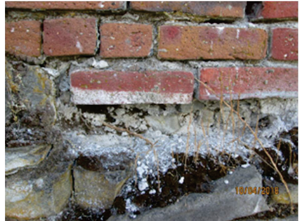
PHOTO 50: A former mortar line at the first brick course indicates that the transition may have been parged to form a water shedding slope.
