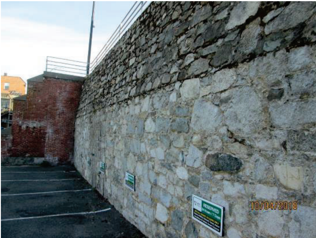
PHOTO 77: General view of the stone retaining wall, showing the upper sloped (battered) section.
