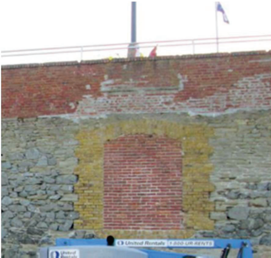
PHOTO 43: Infilled doorway. The red brick may be recycled from the original construction.
