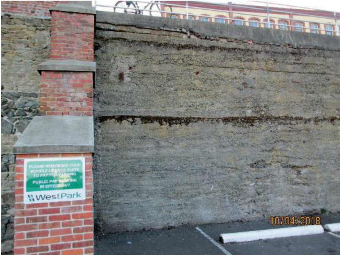
PHOTO 63: The cast in place concrete wall shows a stratification typical of concrete placement technique, common place in the early 20 th century.
