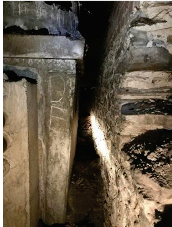
PHOTO 58: The end wall appears to be perpendicular to the warehouse wall.
