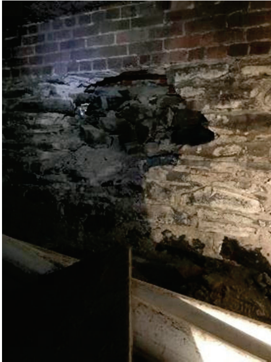
PHOTO 59: A 1.0 x .75 m area of masonry has been removed from the HBC wall. In this location the remaining stone work appears to be 150mm thick.
