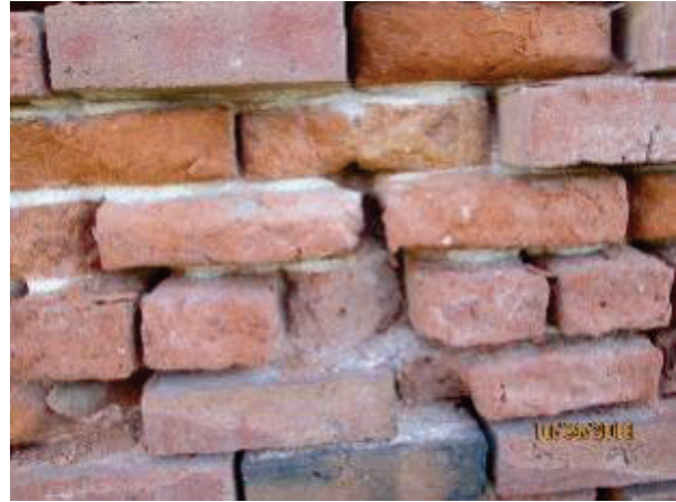
PHOTO 74: Sample area showing different rates of degradation due to variations in the density of the clay brick. Typically, the bricklayers would select the lower fired and duller sounding bricks for the interior surfaces during construction.
