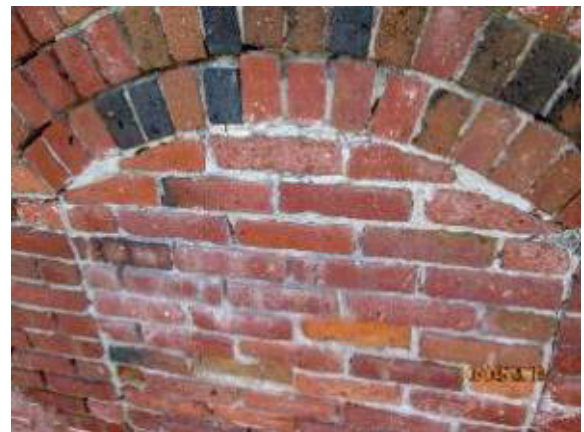
PHOTO 72: Infilled borrowed light window. The opening was likely filled in using recycled bricks,
