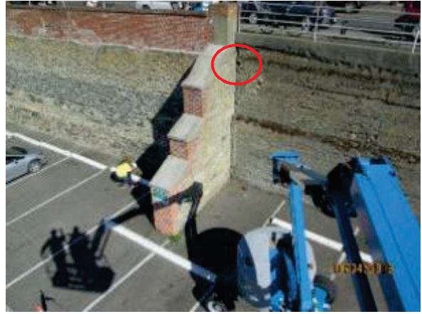
PHOTO 65: A general overview of the section 2 wall and the northerly buttress, repaired in 2013. Highlighted is the small aperture where the void behind section 1 was observed.
