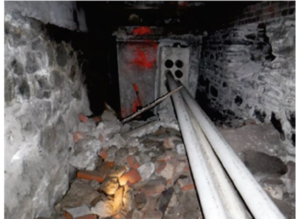
PHOTO 56: Construction debris, possibly from the deconstruction of the warehouse in 1937.
