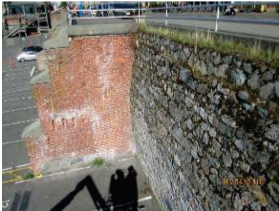
PHOTO 22: The infill brickwork between the Turner Beeton warehouse wall and the rock retaining wall.
