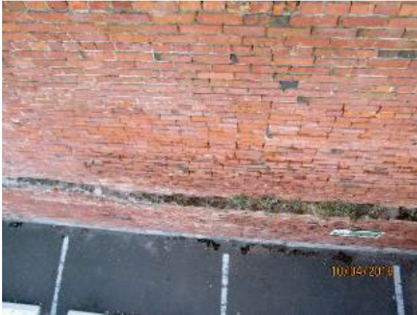
PHOTO 73: An overhead view clearly reveals the mortar loss at the joints and degradation of the exposed brick surfaces.
