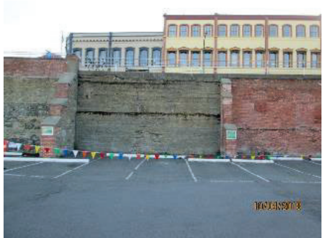
PHOTO3: SECTION 2 Cast in place concrete section formerly part of the wharf access ramp.
