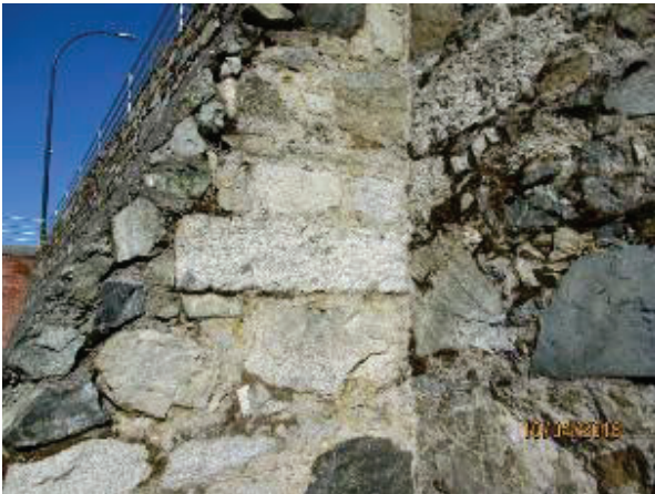
PHOTO 82: Recent repairs to the buttress are evident. Stone has been added to provide a facing guide for the sloped mortar cap.
