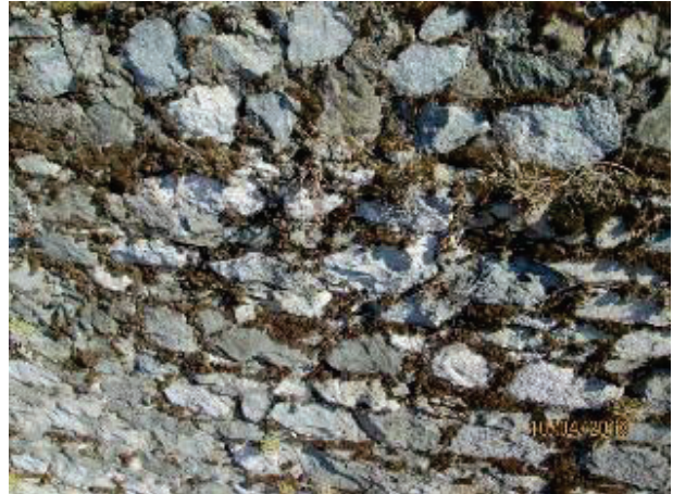
PHOTO 79: Organic growth at the mortar joints.
