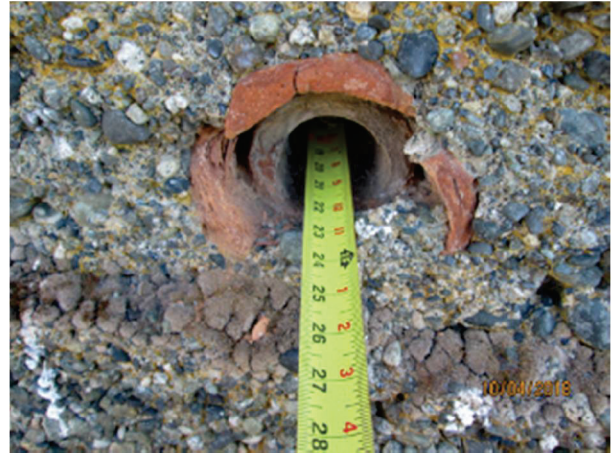
PHOTO 69: Clay drain tile insert.
