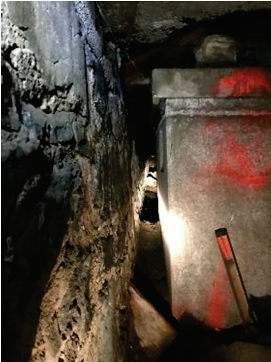
PHOTO 57: A stone masonry end wall appears to align with the end of the warehouse building.
