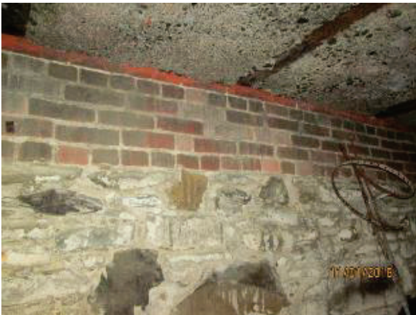
PHOTO 53: The HBC warehouse wall. Mortar jointing has not been subjected to prolonged weathering and was found to be in good condition.
