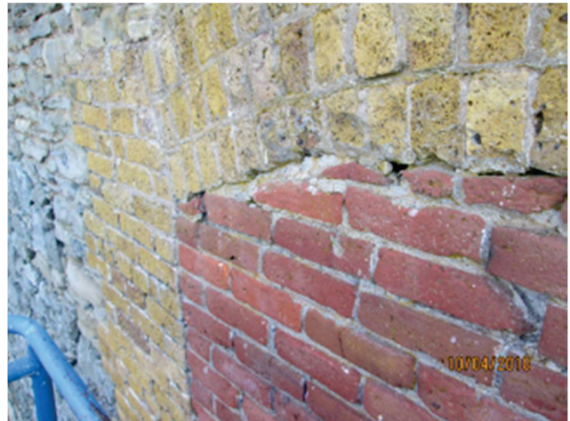
PHOTO 44: Relieving arch in detail. The tan bricks are clearly part of the original construction.
