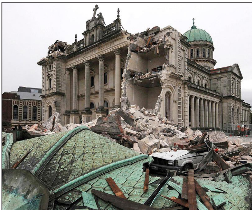
Fig. 4.4: Cathedral of the Blessed Sacrament partially collapsed in the February 2011 Christchurch earthquake. After eight years of debate and the site left in disarray, it was decided in 2019 to demolish the remaining sections of the Category I heritage-listed structure from 1905. (Source: New Zealand Press Association, David Wethey)
