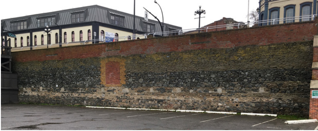
Western retaining wall and first floor interior elevation of the 1858 HBC Warehouse on Wharf Street, Victoria.
